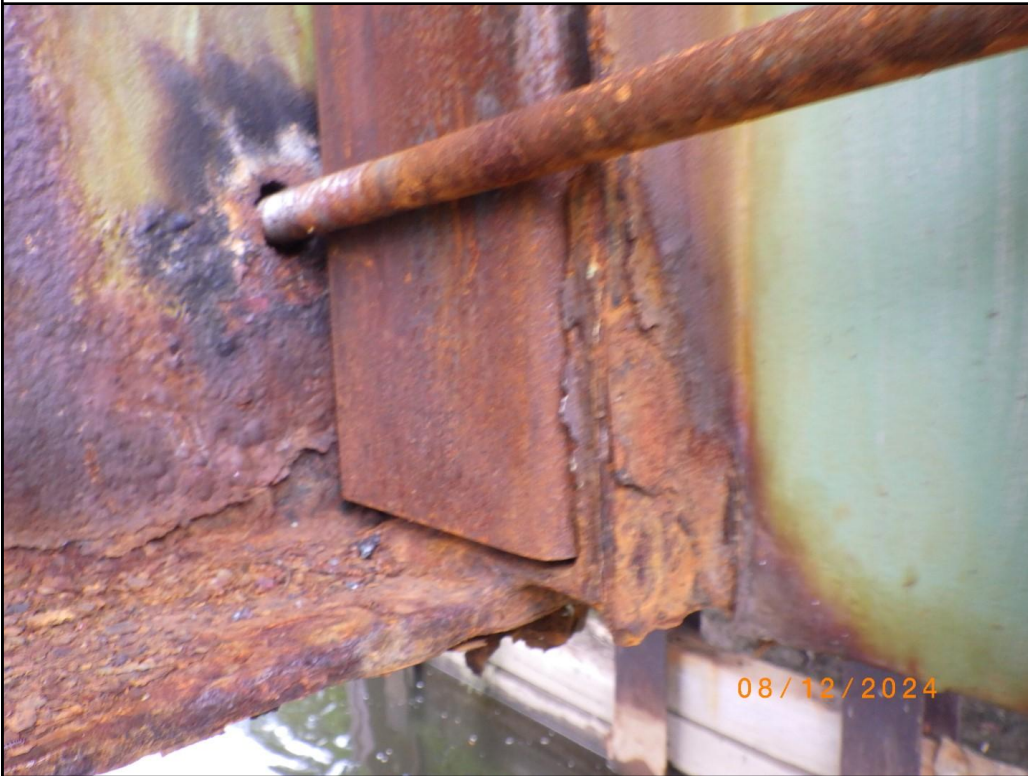
Special Emphasis Detail- Railing Bottom Flange Welds.JPG
